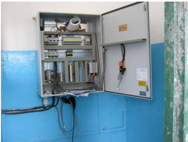
Fig. 3: Monitoring and control unit
