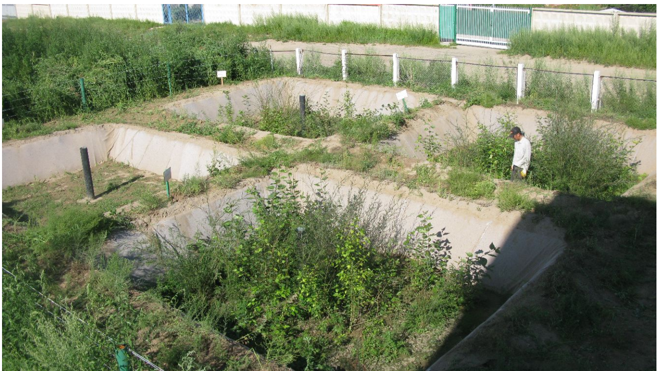
Fig. 3: Wastewater treatment basins
